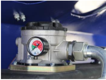
Filter Housing with Pressure Gauge
