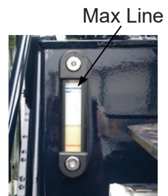
Fig. 7.4 Hydraulic Tank Site Gauge
