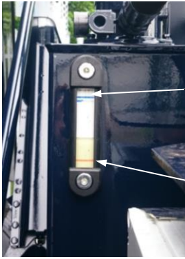
Fig 1.1. Hydraulic Tank Site Gauge
